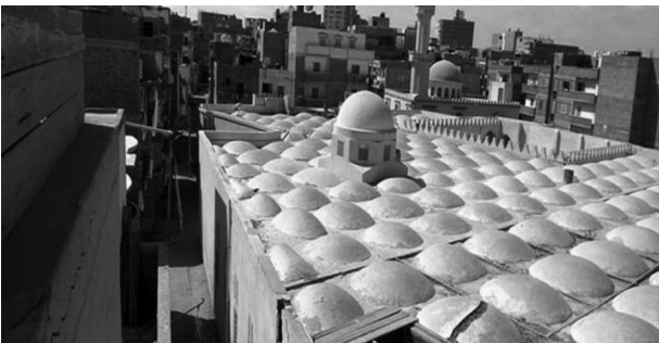
Figure 22. Roof of Zaghoul Mosque, showing the unique architectural style and poor condition of domes (Abudeif and Hefny 2018).
